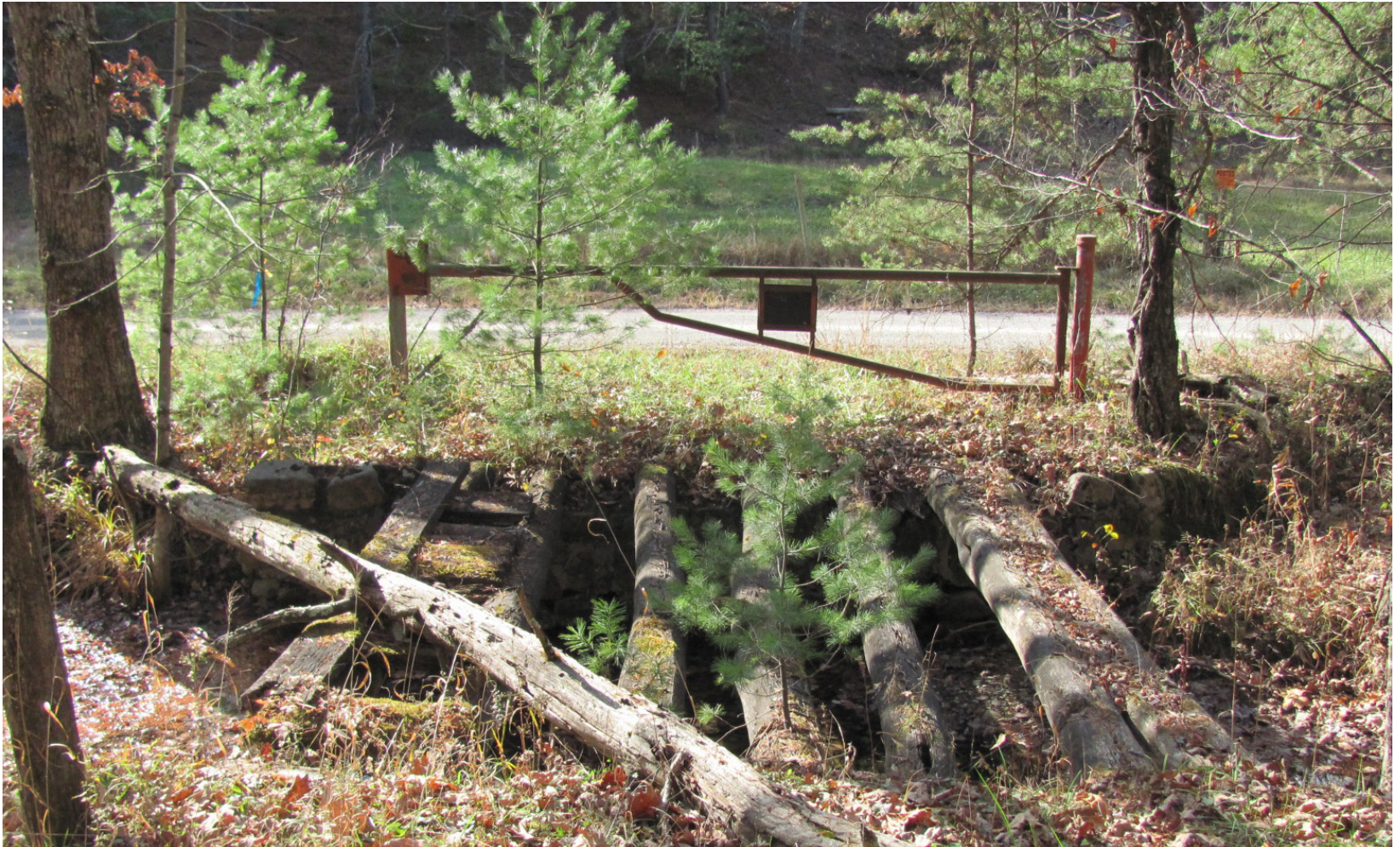
Remains of a bridge on White Sulphur Spring Road.
